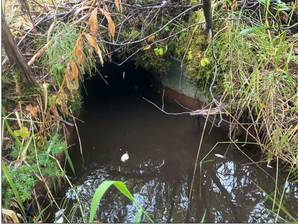
Figure 2.—Stream channel at waypoint 1245.
